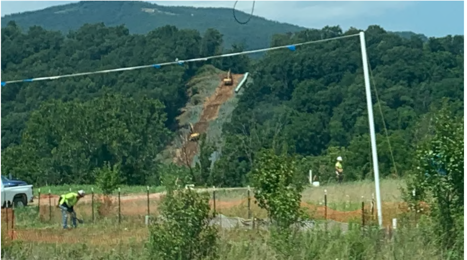
The Mountain Valley Pipeline near Elliston in Montgomery County. Photo by Kevin Myatt.
