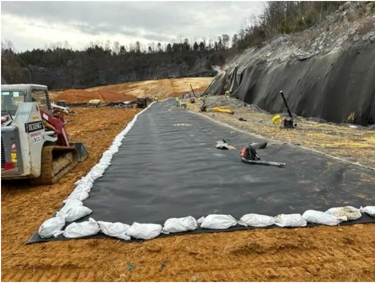
Geomembrane (black panel) that will wrap around the sidewall gas collection system, providing a seal that prevents the release of odorous gases. Courtesy of city of Bristol.
