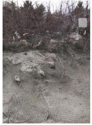
Shotcrete applied on quarry wall to seal cracks in rock that can convey odorous gases. Courtesy of
