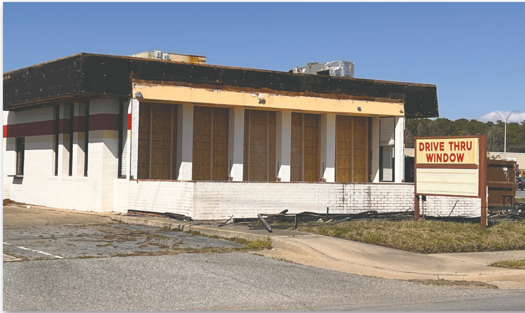
Work is underway on Armory Drive at the former Golden Skillet site, which will become a new Dunkin' Donuts location, expected to open this summer.
