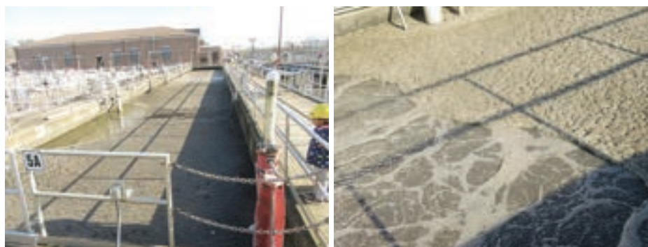
This wastewater is undergoing secondary or biological treatment using bacteria.
