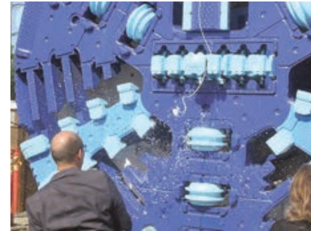
On July 14, Alexandria Mayor Justin Wilson christened Hazel by breaking a bottle of treated wastewater on the machine.
