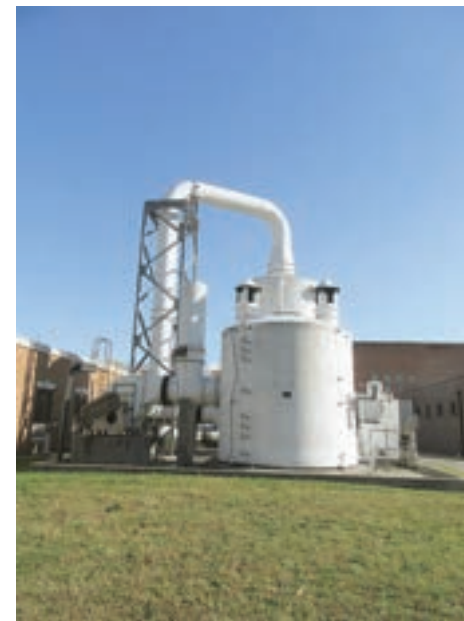
A biotower, odor control technology.
