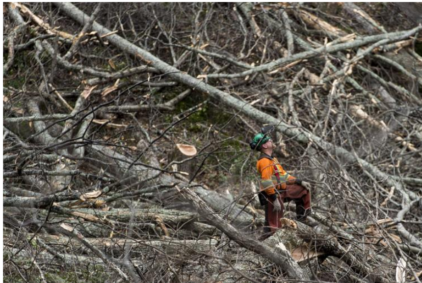
In this March 2018 file photo, a swath of trees lays fallen at Wintergreen after being cut by crews clearing the route for the Atlantic Coast Pipeline. The News & Advance file
