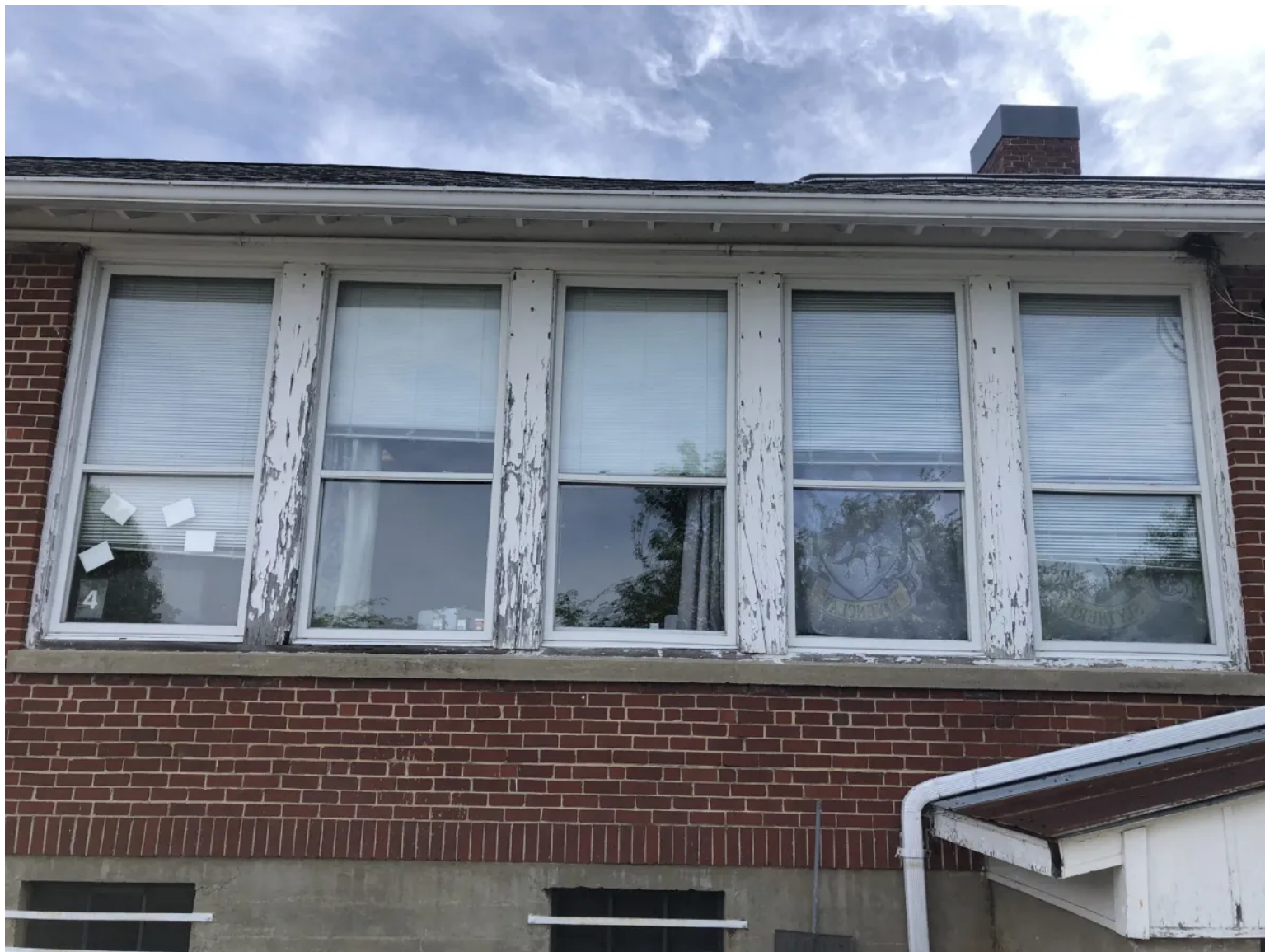
The exterior of Highland View Elementary in Bristol, a school declared "functionally obsolete" in 2011 but still in use. Courtesy of Bristol Public Schools.
