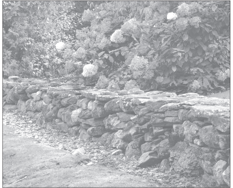
This new dry stacked stone wall has a base of crushed stone and flat rocks on top, giving it stability and a more carefully planned appearance.
