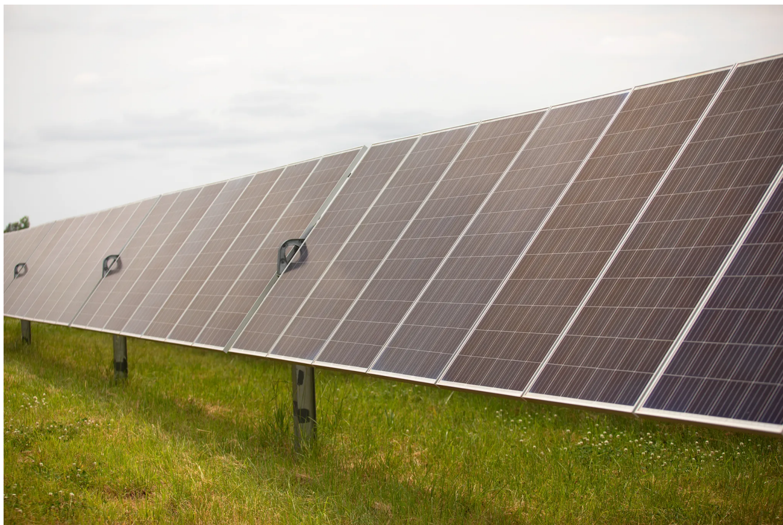
A Dominion Energy solar farm in Powhatan County. Courtesy of Dominion Energy.
