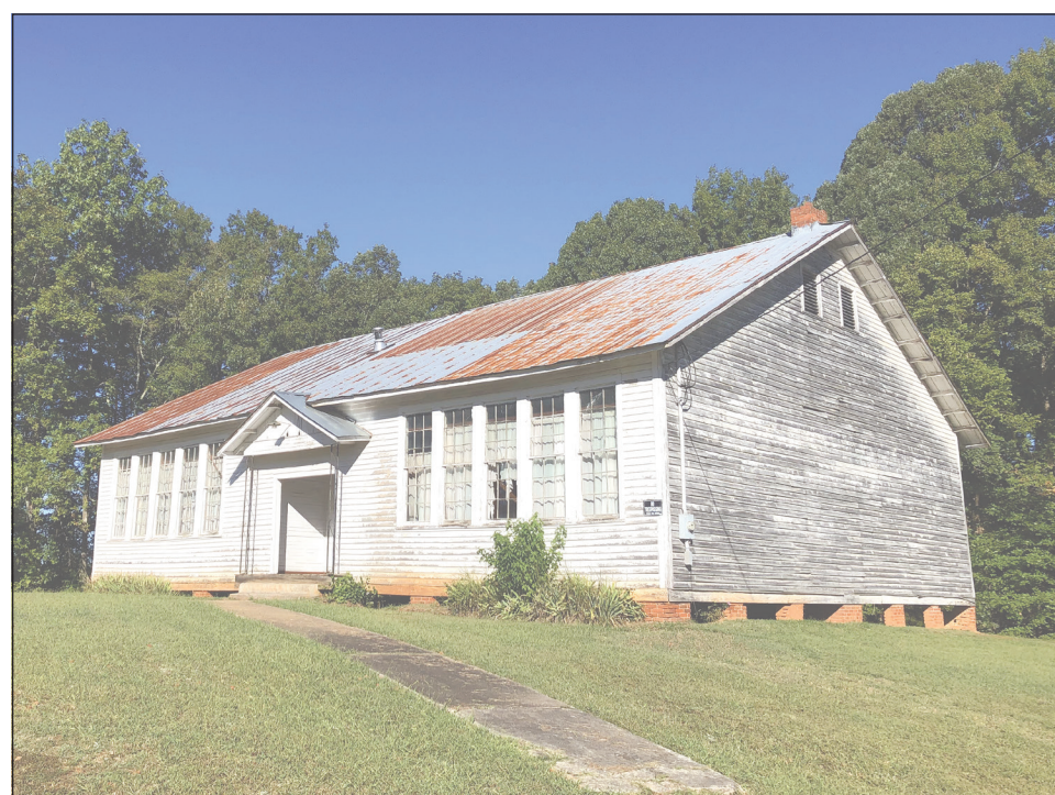
The former Salem School in Red Oak is in the process of being restored.
