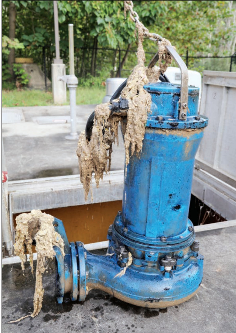
Disinfectant wipes can gum up the machinery at the county's wastewater treatment plants. These wipes were removed from a sewage pumping station; the blue machine is a submersible pump.
