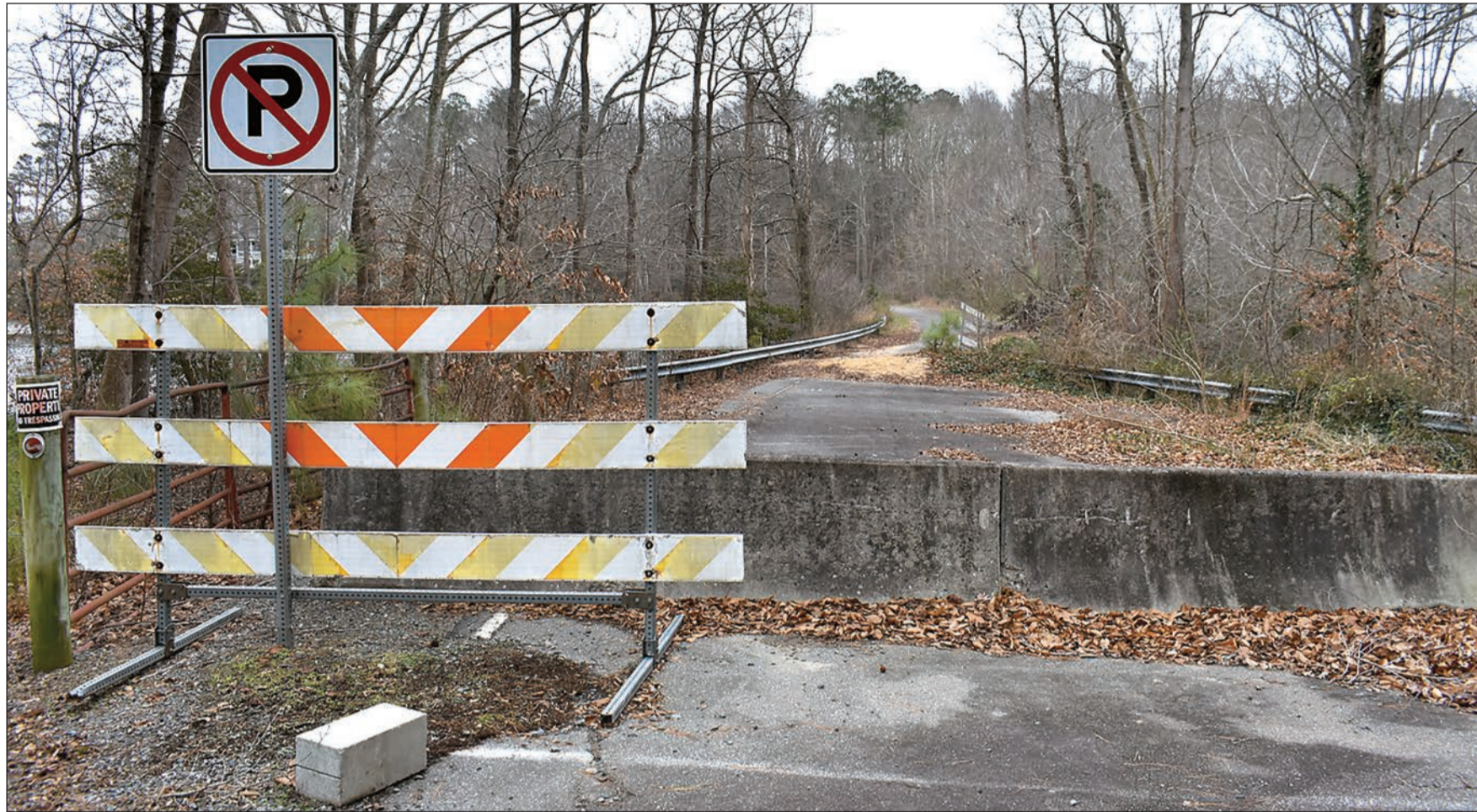
Route 629 over Healy's Mill Pond near Hartfield has been closed since 2006 as VDOT and the Middlesex County Board of Supervisors were then unable to come to an agreement as to who was responsible for funding repairs to the dam and road over the mill pond. GPS directional information has continued for 15 years to send visitors down the dead-end road, causing a hardship to the Piankatank River Golf Club and others located on the road.
