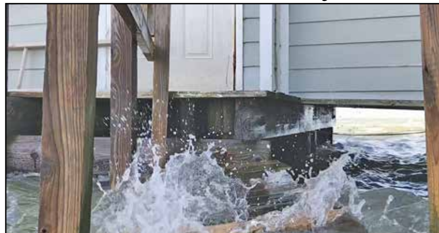
Water laps at the Chesapeake Bay Foundation's education center on Fox Island. Rising sea level has led to a decision to close the facility. (Jeremy Cox)
