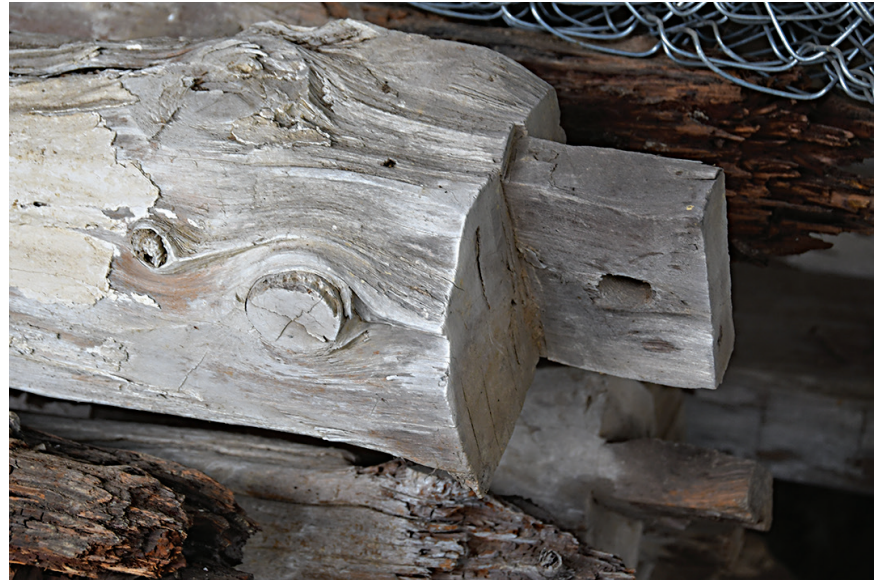
A tenon shaped on a cedar tree once fit into a mortise as part of a building frame.
